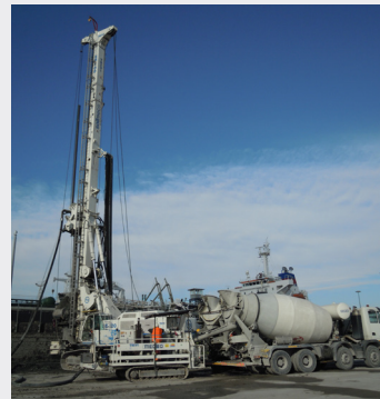
Construction of an impermeable barrier using cased secant piles. Casting of Solidur® Erdbeton plastic concrete
