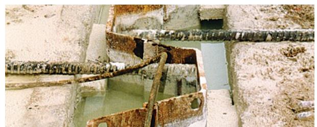
Trench sheet paced inside the barrier with Solidur® still in the liquid state
