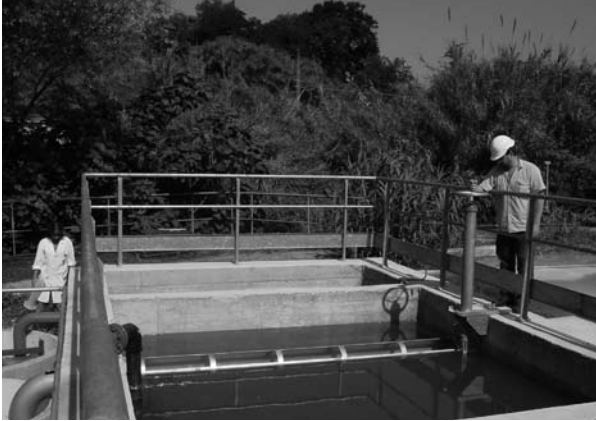
Water treatment system
