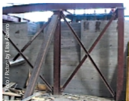
Blocco del mulino: superfici scasserate Surface of the mill pier after the forms have been removed
